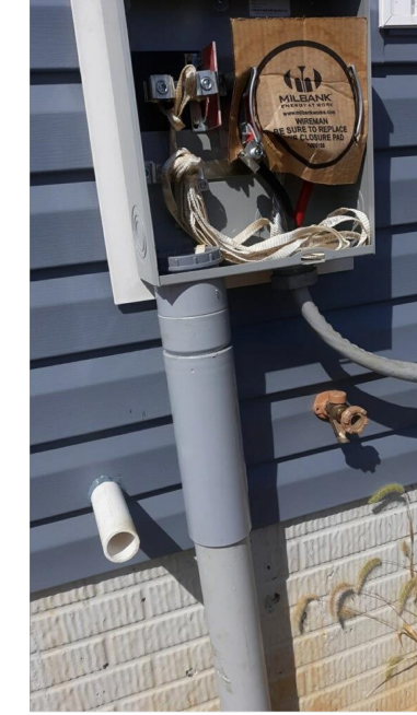
Inside of Meter Pan with mule tape/pull string
