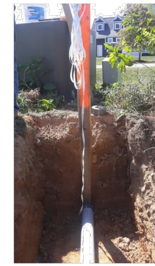
Capped off end at DPL equipment
