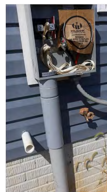
Inside of Meter Pan with mule tape/pull string
