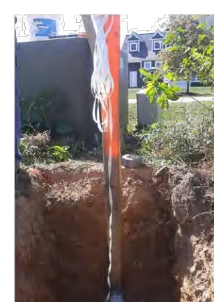
Capped off end at DPL equipment
