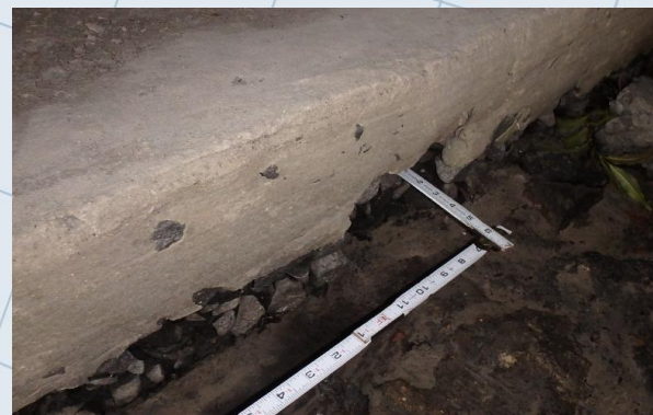
Scour exposing the culvert footer. Note the deep abrasion in the culvert footer as shown by the ruler probing it.
